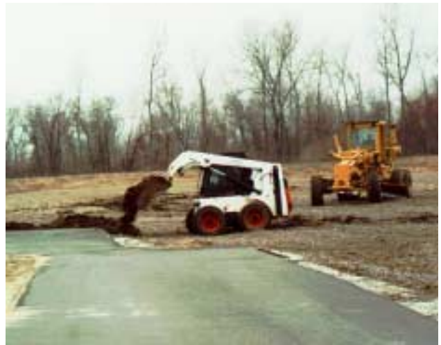
This Bobcat was used for further smoothing the dirt along the edges of the asphalt.
